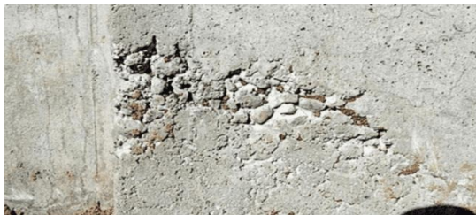
Figure 3.1 Image of Voids and Honeycomb
