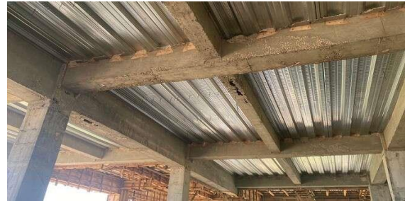
Figure 3.3 Documentation of Deformed Beam
