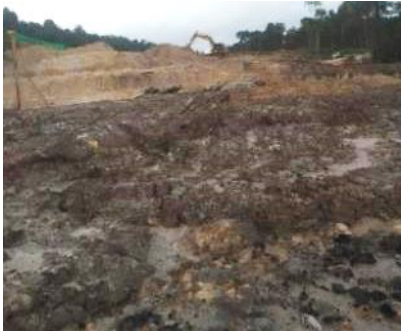
Figure 4. 13 Work Areas Unusable (Source: Personal Documents, 2023)
