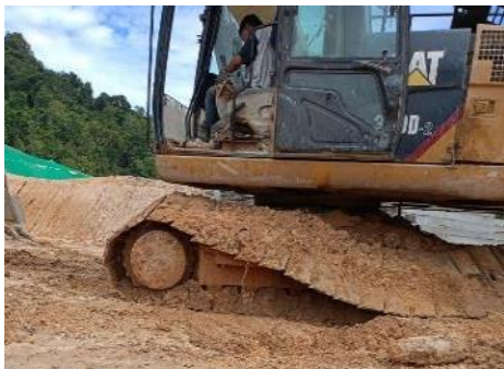
Figure 4. 14 Machine Damage (Source: Personal Documents, 2023)
